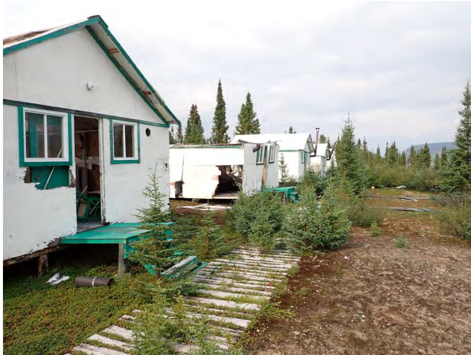
Figure 10.14: View towards the north-northeast of dilapidated cabins at the former Chambeaux outfitting camp.
